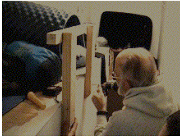
Figure 6: Adding a makeshift guard rail to an upper bunk [MDRS-5]
